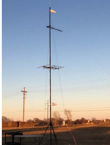
Figure 9: Base Station Mast and Antennas
